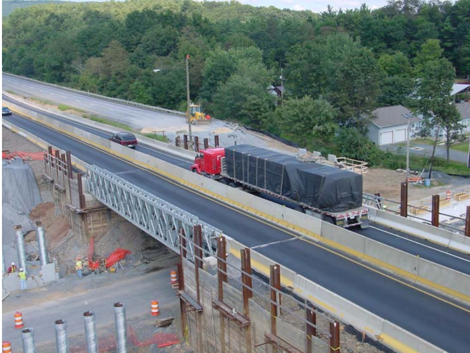
ACROW 700XS BRIDGE ON INTERSTATE HIGHWAY 81 PENNSYLVANIA DEPT. OF TRANS. NEAR HARRISBURG, PENNSYLVANIA
