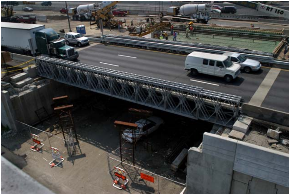
ACROW 700XS BRIDGE ON INTERSTATE HIGHWAY 95 CONNECTICUT DEPT. OF TRANS. NEAR NEW YORK CITY, NEW YORK
